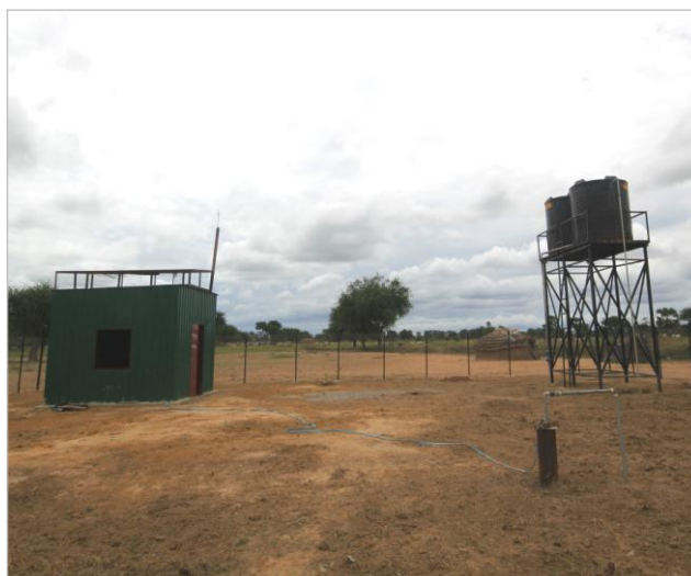
Figure 15: Inside Pandit Water Yard
