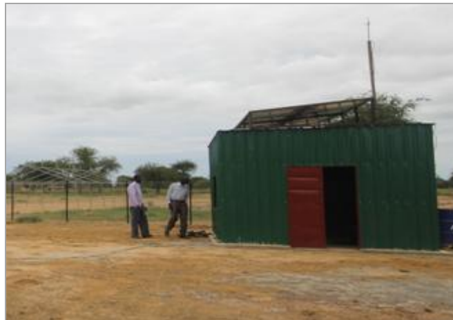
Figure 12: Solar panels at Pandit Water Yard
